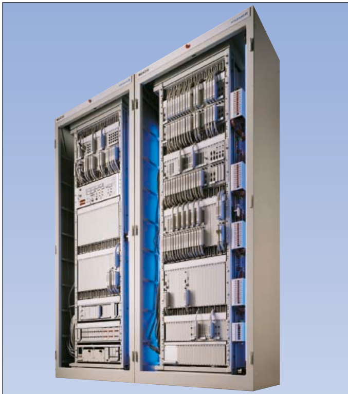
ME 4012 system cubicle with digital turbine controller and digital turbine protection
