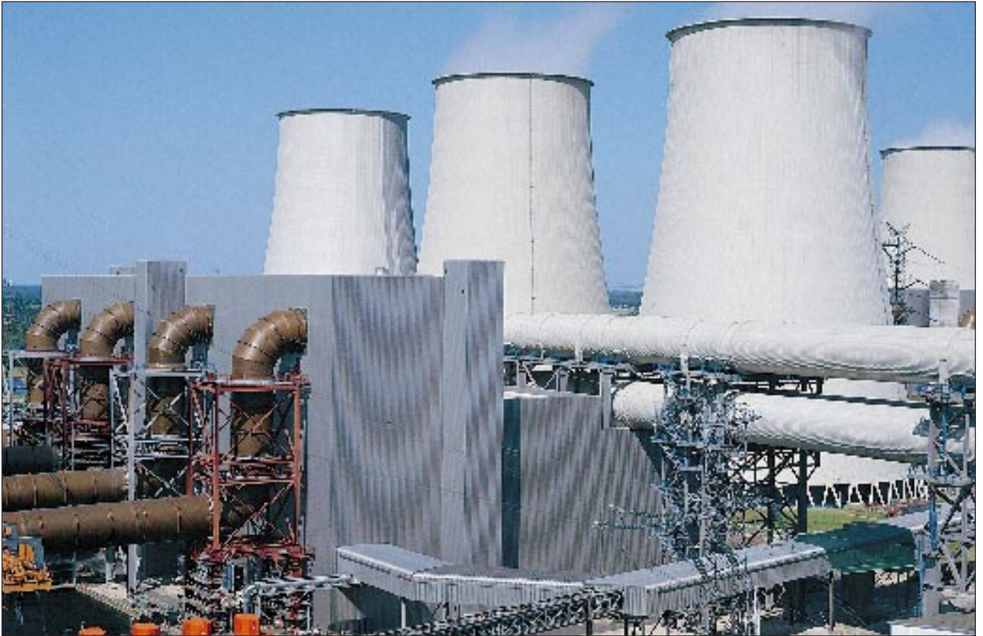
REA Braunkohlekraftwerk / Coal power station (Flue gas desulfurization)
