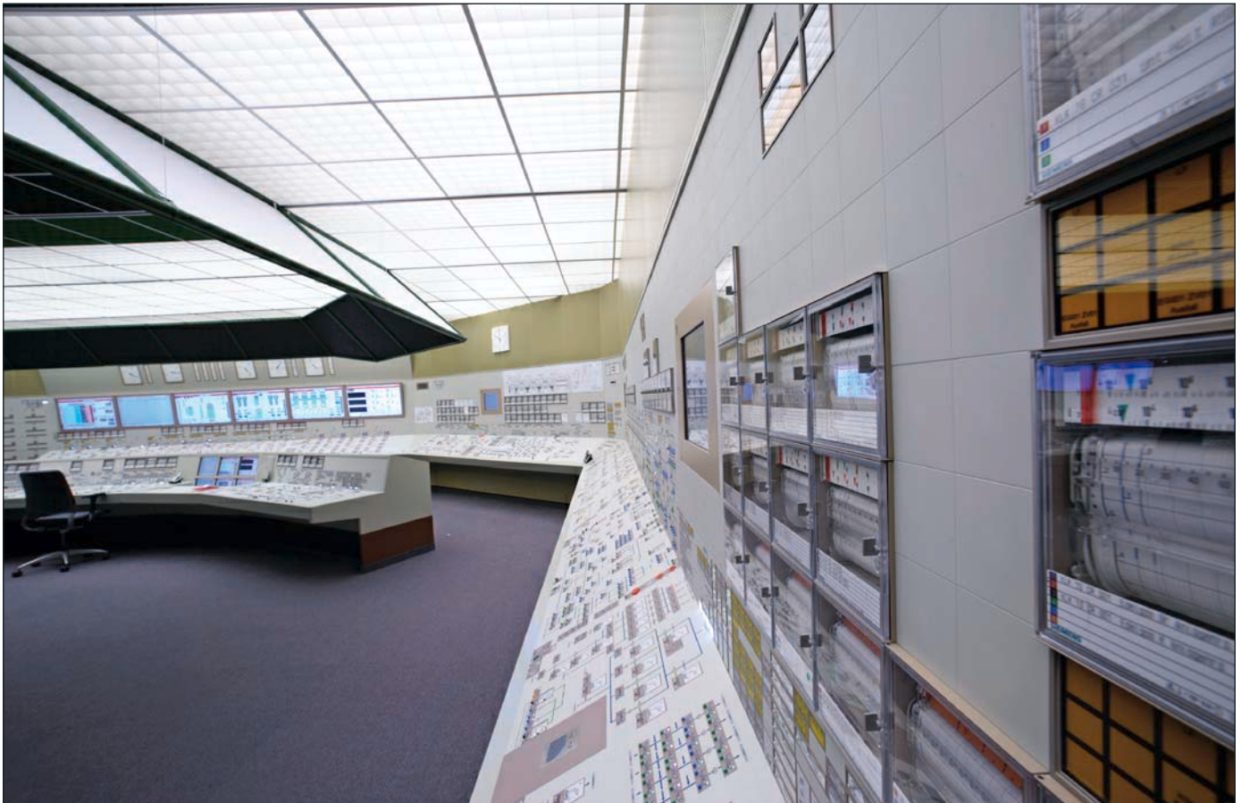
Kraftwerkswarte / Power Plant Control Room
